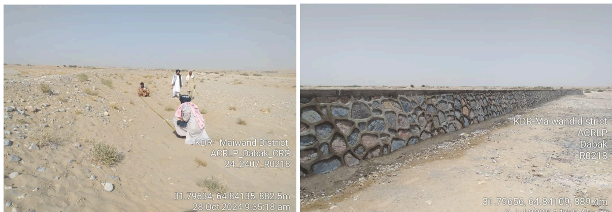
Before and After pictures of protection wall construction for Dabak CRG in Maiwand District , July 2025 @FP/CHA
