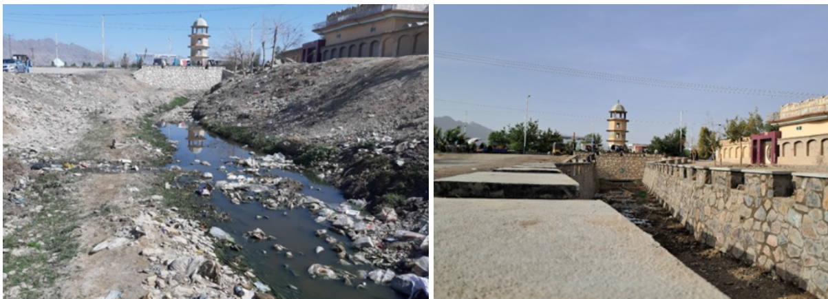
Before and after photos of a surface water and flood control canal in Gozar #4, District #1, Kandahar City on 19 June 2025 @UNOPS
