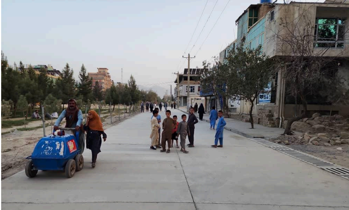
Street paved with plum concrete and handed over to the community in Gozar #6, District #12, Kabul City, on 25 August 2025 @UNOPS
