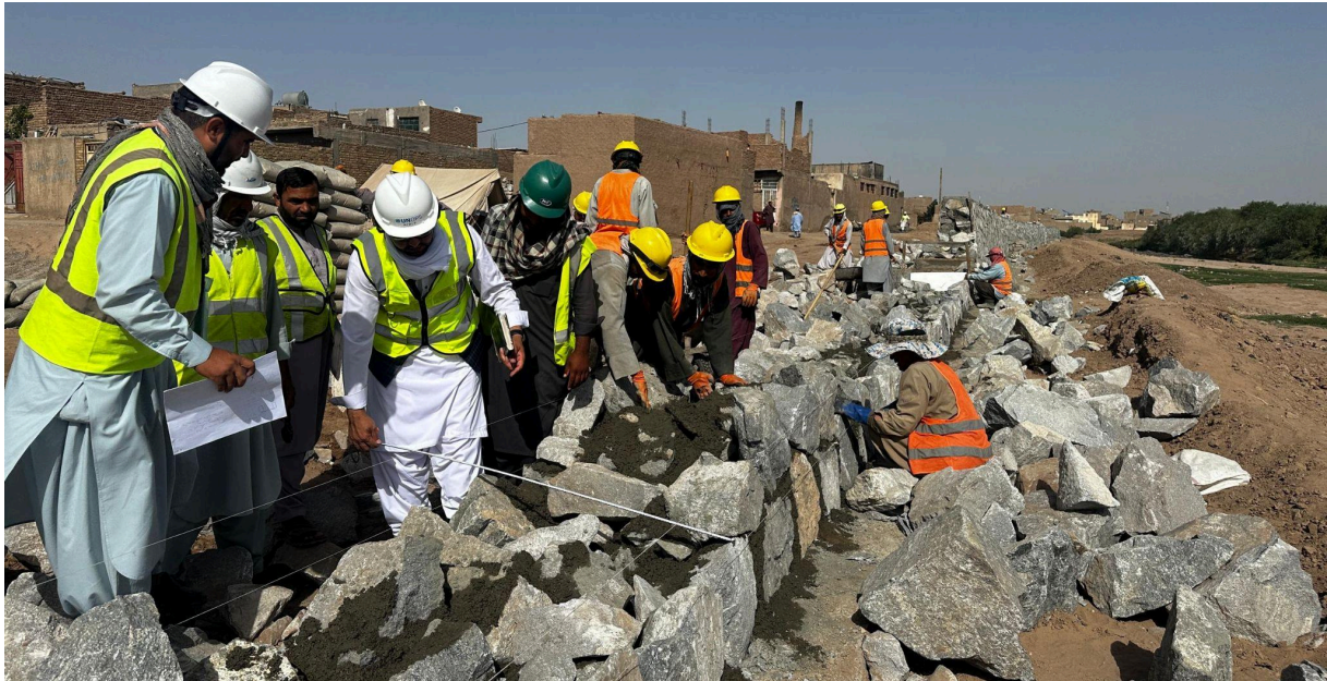
Field supervision of UNOPS Construction Management Engineer from a flood protection wall project in District #10, Herat City on 27 August 2025 @UNOPS
