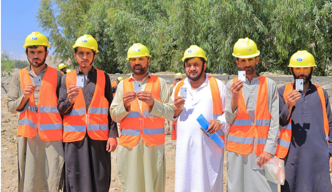
A group of returnees working at a construction site for a protection wall in Jalalabad, June 2025 @UNOPS/Rafiullah Hemat
