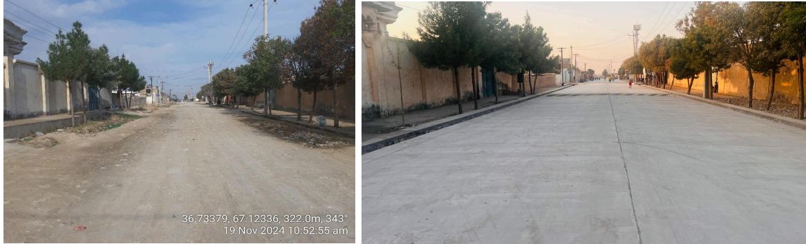
Street paved with plum concrete and handed over to the community in Gozar #5, District #8, Mazar City on 17 August 2025 @UNOPS
